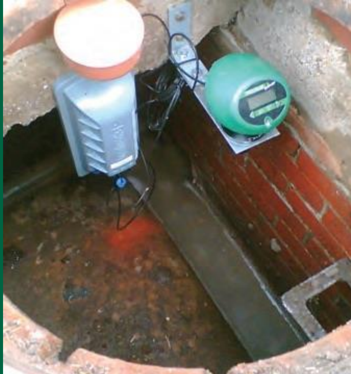
Ultrasonic water level meter at Sewage junction(CSO)
